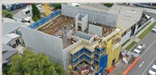
Double-storey precast panels providing a safe construction method when building boundary to boundary.
