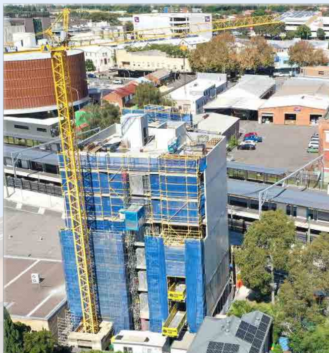
Site logistics solution at building rear: Tower crane, personnel hoist, and retractable loading platforms.
