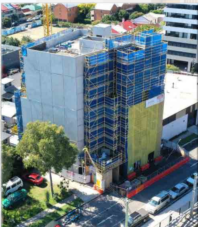
Station Street site logistics solution: Hoarding permit, work zone, ROP/lane closure and redirection.
